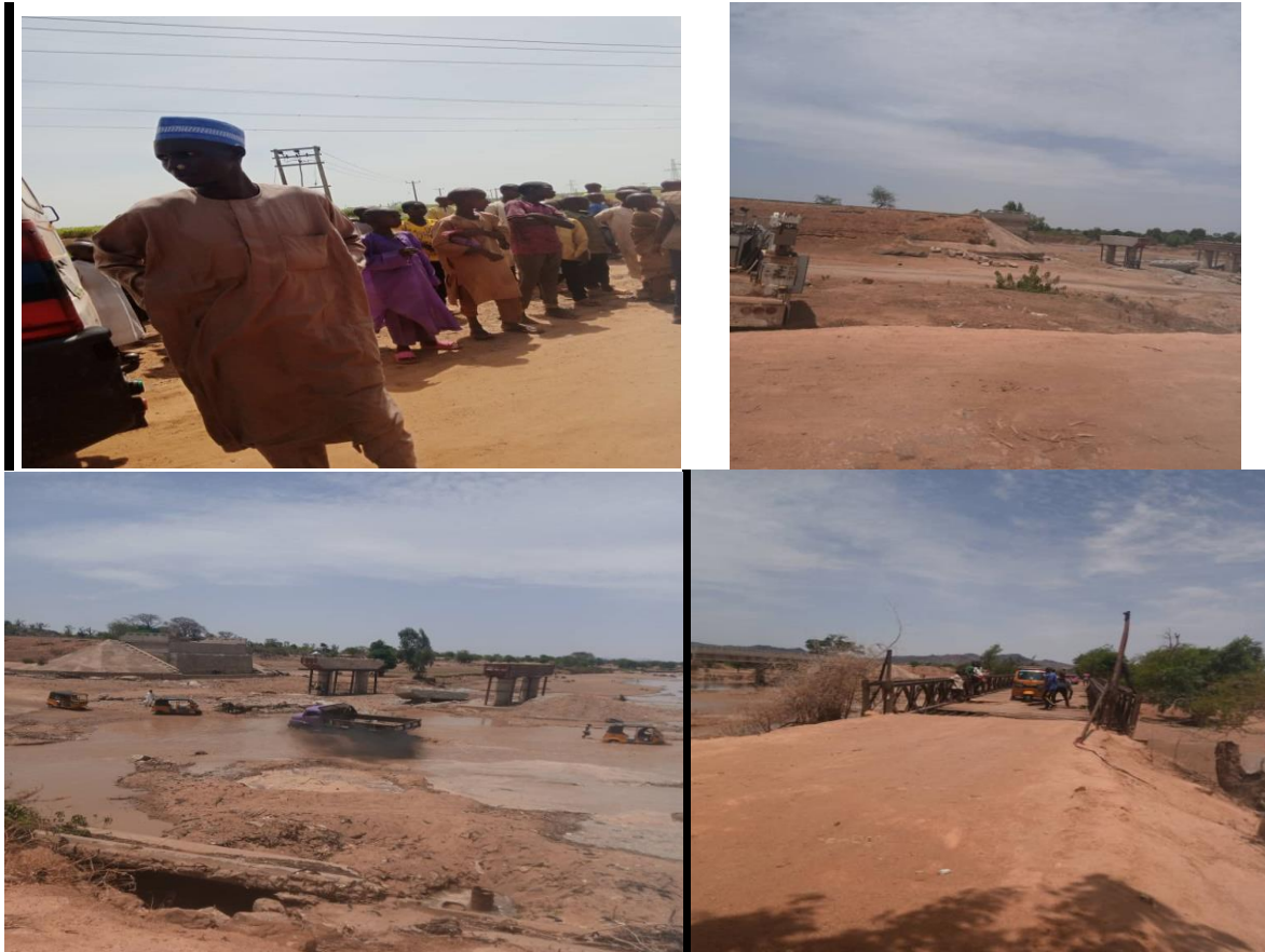
Need assessment in North East- Damages of roads by Boko Haram (Yola to Maiduguri)
